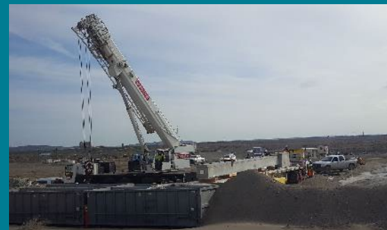
Workers use a crane to place a large item into a Super Cell for disposal.
